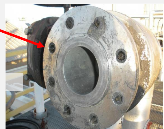
BV Bolting Failure
