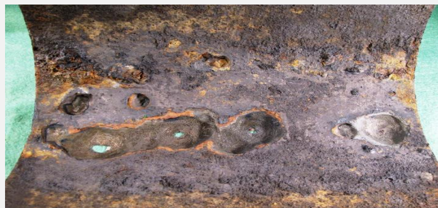
Close-Up of Pitting
