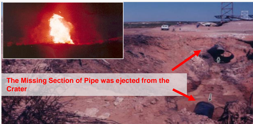
Gas Pipeline Failure – New Mexico 2000
