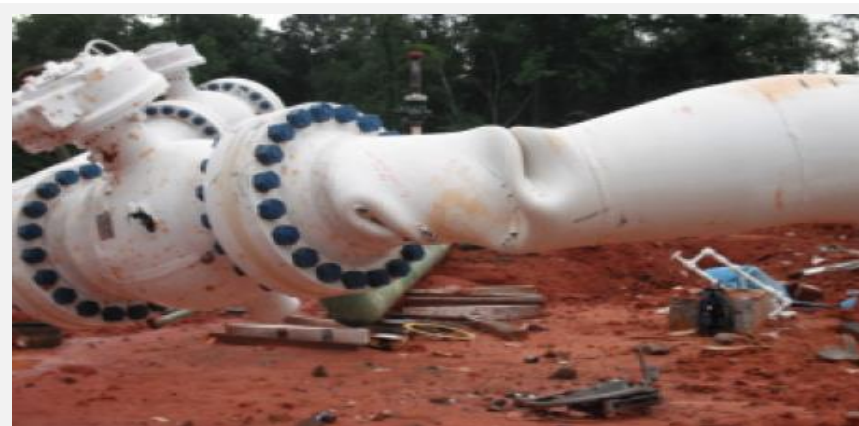
Resulting Hydrotest Failure
