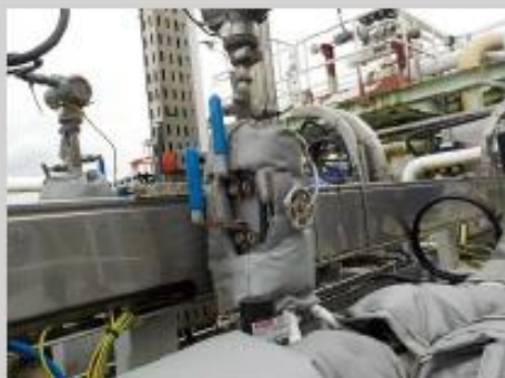
DL4 - Partially under insulated jacket.
