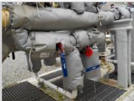
DL2 - Under insulated jackets.
