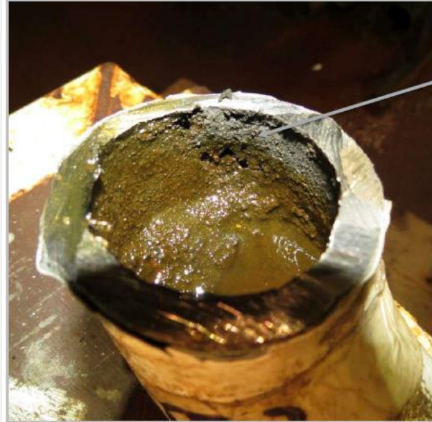
Failure Site and Sludge Below.
