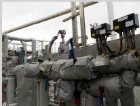
DL5 - Under insulated jackets.
