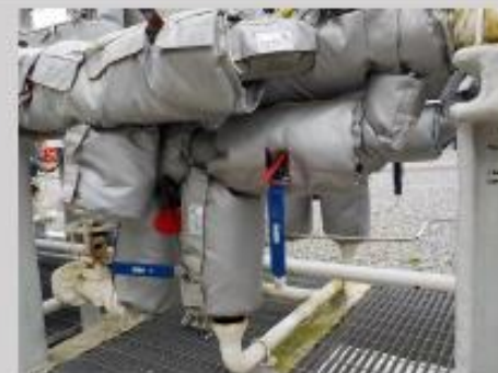
DL6 - Under insulated jackets.
