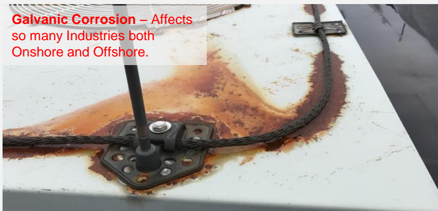
Safety Earthing – Typ. Galvanic Corrosion
