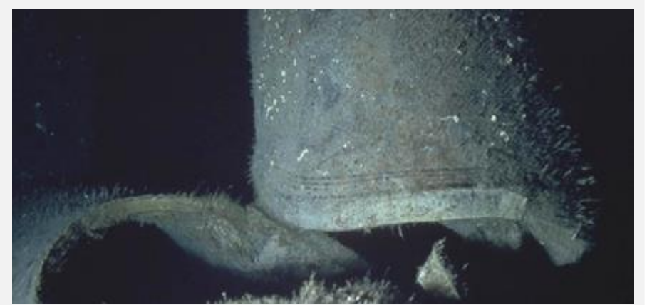
Subsea Structural Failure
