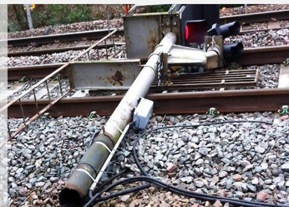
Newbury Railway – Corroded Signal Base
