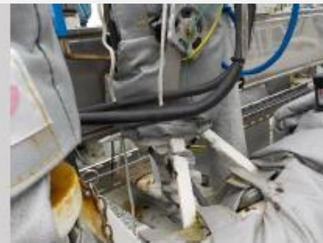
DL3 - Partially under insulated jackets.
