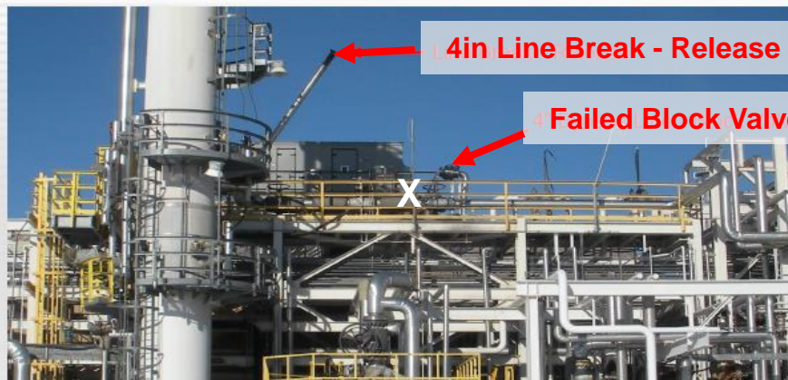
Sour Gas Leak 2011
