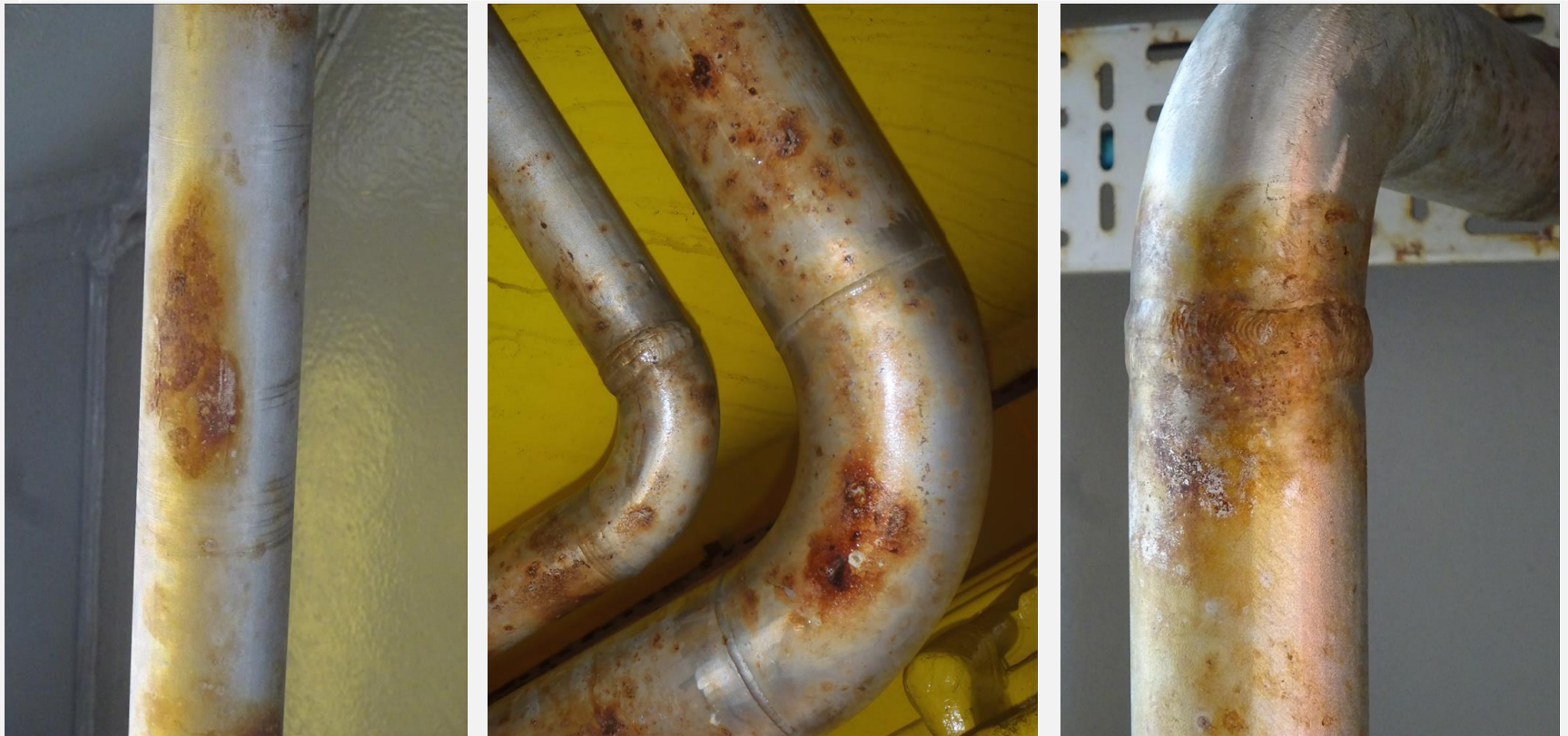
Poor Fabrication / Material Selection Practices – Uncoated 316L in Marine Environment
