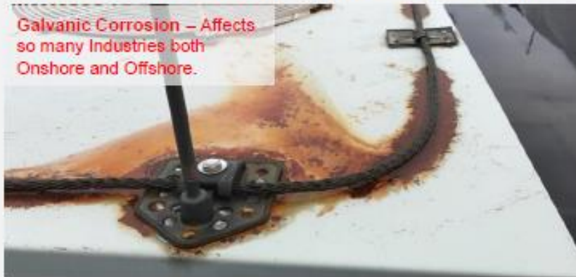
Safety Earthing – Typ. Galvanic Corrosion
