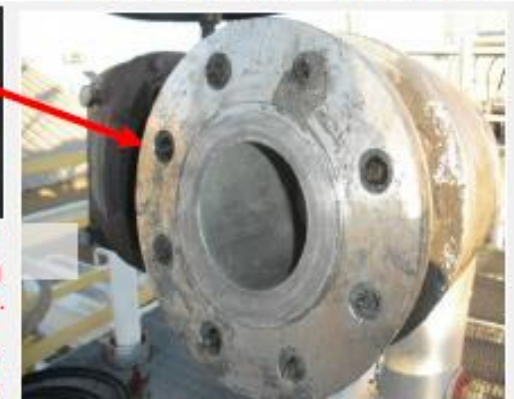
BV Bolting Failure
