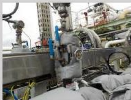
DL4 - Partially under insulated jacket.
