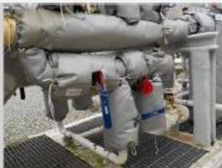
DL2 - Under insulated jackets.
