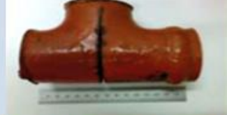
H2 Induced Crack
