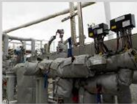
DL5 - Under insulated jackets.
