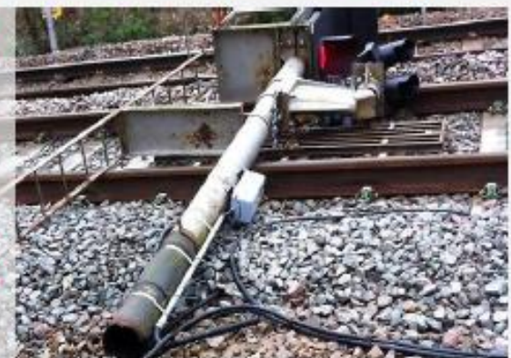
Newbury Railway – Corroded Signal Base
