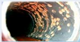
Sour Fluids Pitting
