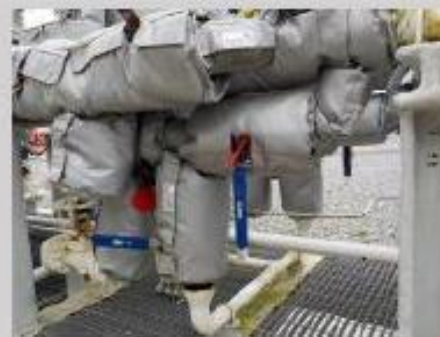
DL6 - Under insulated jackets.
