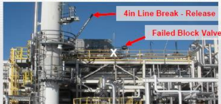
Sour Gas Leak 2011
