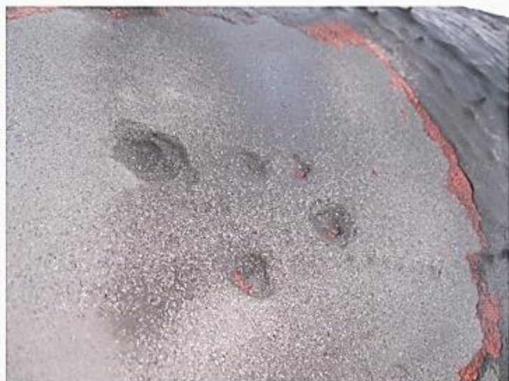
ILI 1. Condition prior to repair (MFL1)
