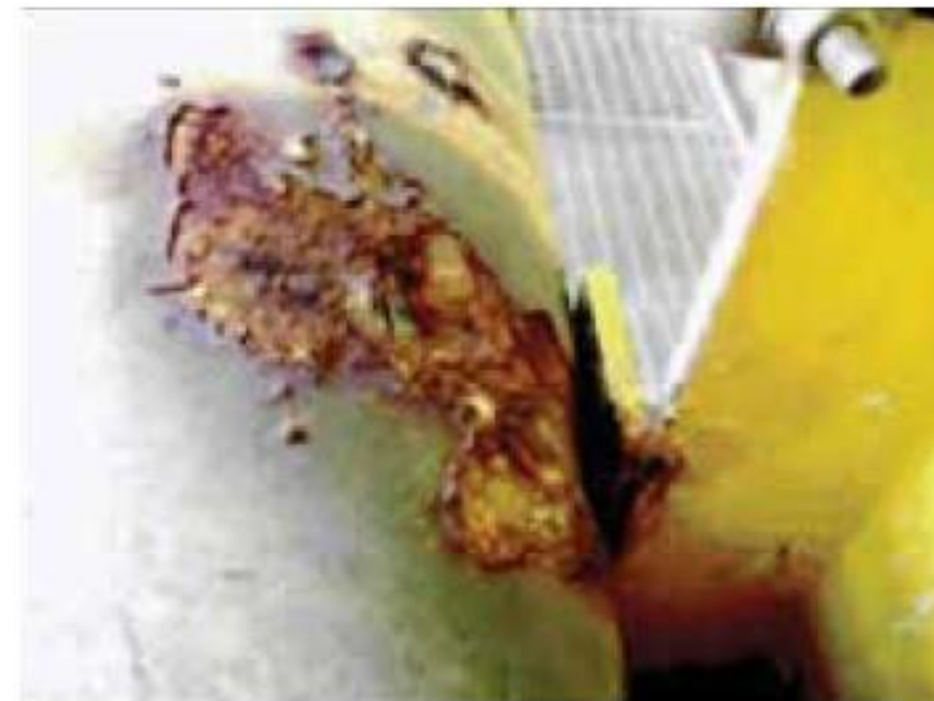
External corrosion of a pipe at a pipe support. Both the pipe and support are corroding at the crevice formed between the two. The coating is also breaking back as it under rusts the crevice at the edge (Ref: Guidance for corrosion management in oil and gas production and processing, second edition, HSE & Energy Institute)
