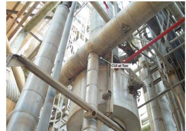
Tee in a 1000 psig ethylene line BEFORE insulation removal (API 571)
