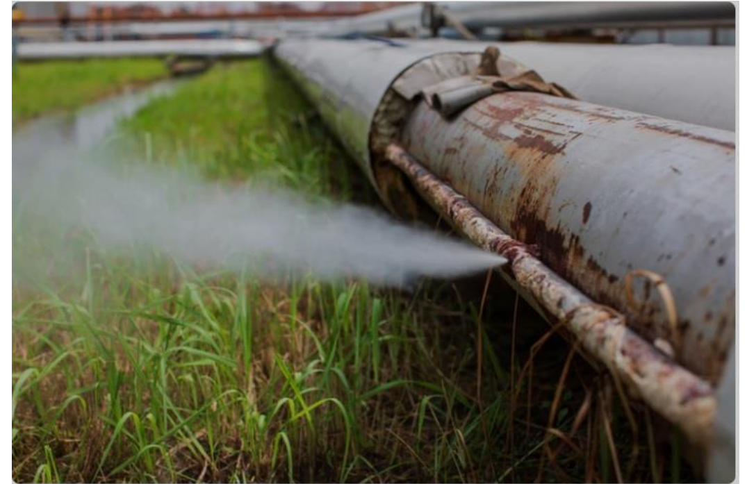
CUI can take the form of localized external corrosion in carbon and low-alloy steels, external stress corrosion cracking or pitting in austenitic and duplex stainless steel ( www.offshore-mag.com )
