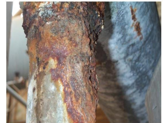
Tee in a 1000 psig ethylene line AFTER insulation removal (API 571)
