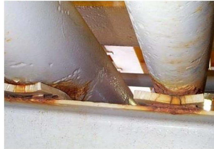
Rubber pads accelerate crevice corrosion www.stoprust.com
