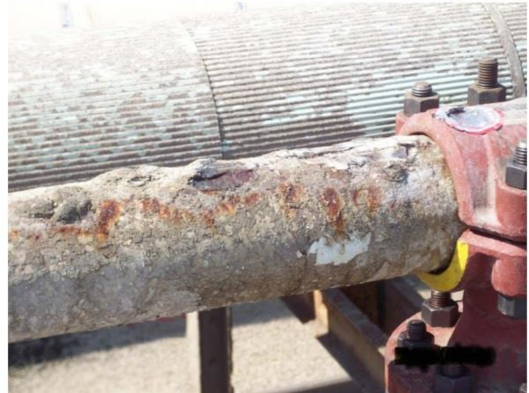
Atmospheric Corrosion of an LPG line in close proximity to a cooling tower (API 571)
