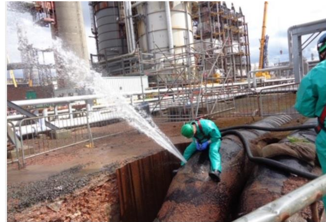
42 Inch cooling water line leak suffered from severe external corrosion ( www.metalytespipework.com )
