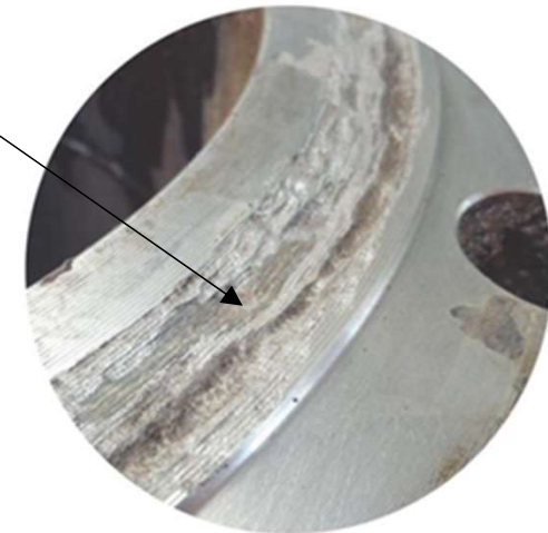
Flange face corrosion
