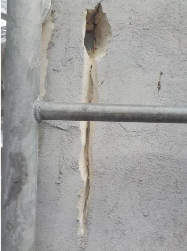
Prepared crack in LWC on vessel skirt
