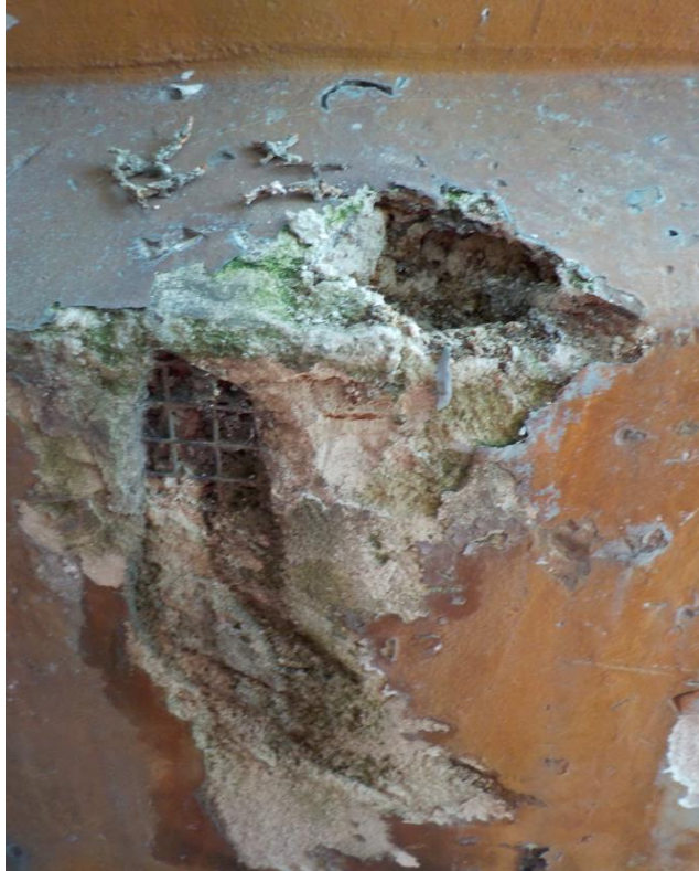
Failed LWC on vessel skirt
