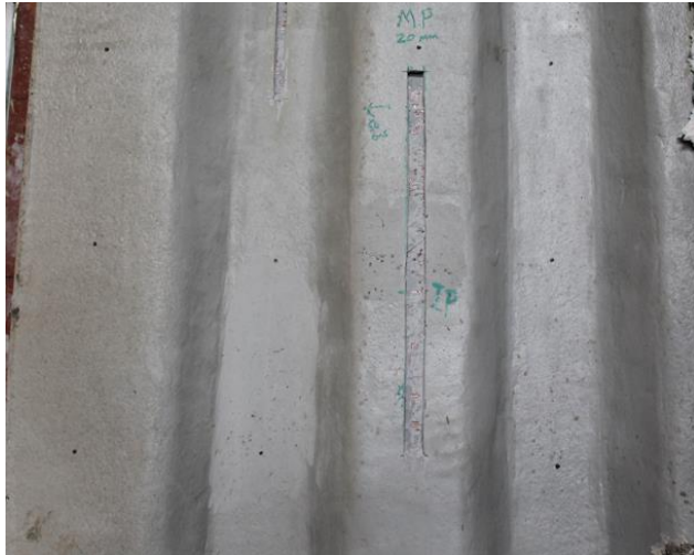
20mm wide 'crack' to steel surface
