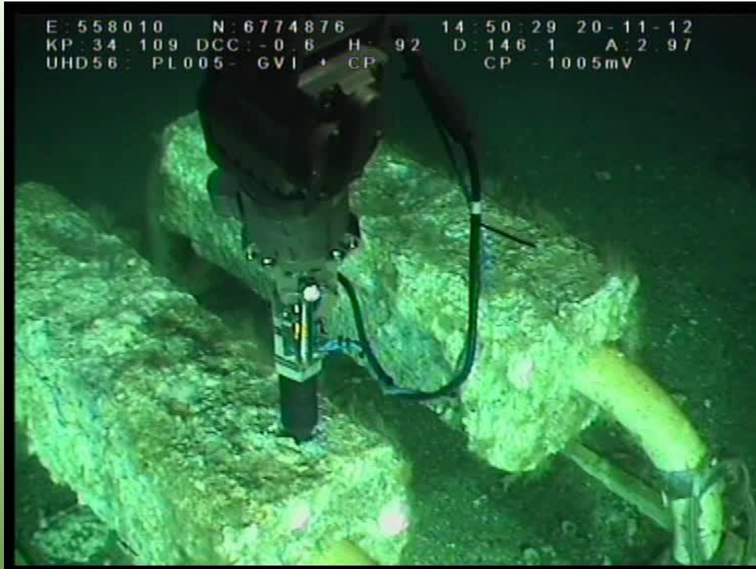
Build-up of Al(OH) 2 on Anode Surface
