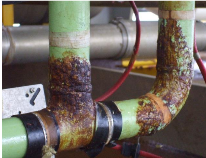
2" gas crossover line
