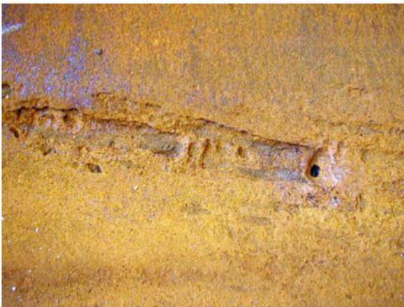
Localised internal corrosion of carbon steel
