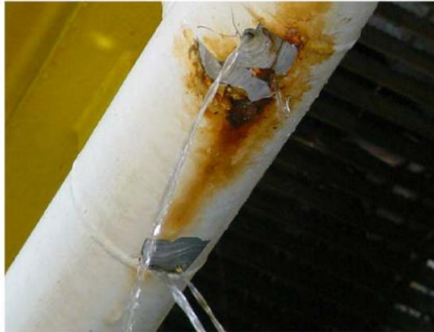
Pitting corrosion of stainless steel pipe carrying seawater
