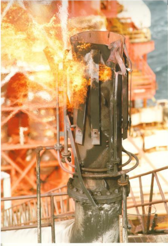
Flare tip – high temperature damage potential
