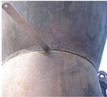
High temperature damage of flare tip
