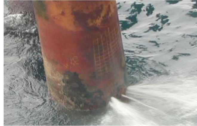
Seawater corrosion of steel platform leg protected by coating
