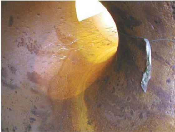
General internal corrosion of carbon steel assisted by flow
