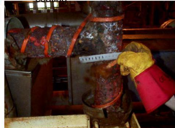
Corrosion under insulation
