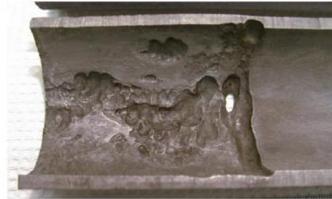
CO_2 corrosion in production tubing
