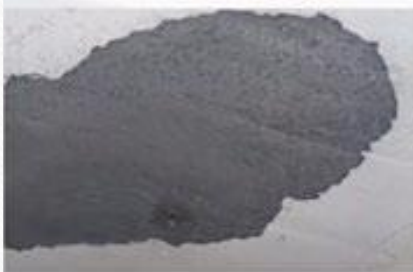
Corrosion pit: depth approximate 0.7mm
