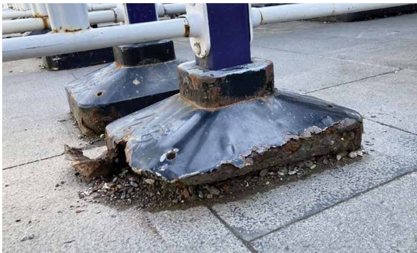
Photo: Structural Corrosion of Pedestrian Barriers, Observed in Xi'an China - October 2024.
