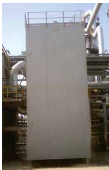
Figure 1: Cold Box Heat Exchanger Unit in A Natural Gas Liquefaction Process Plant.
