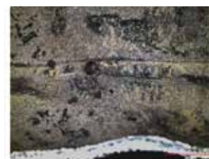
Figure 10: Pitting and Weld Corrosion of a C-276 Heat Exchanger Tube.
