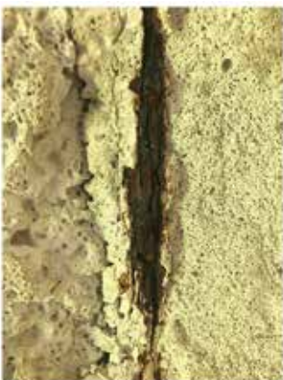
Figure 5: Corrosion in RAAC Seen After a Spall Due to Probable Moisture Ingress Due to a Humid Internal Environment (CPT).
