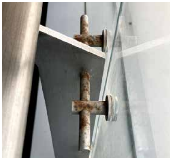
Photo: Atmospheric Corrosion Observed to Hotel Balcony Fixing in Suzhou Anhui, China.
