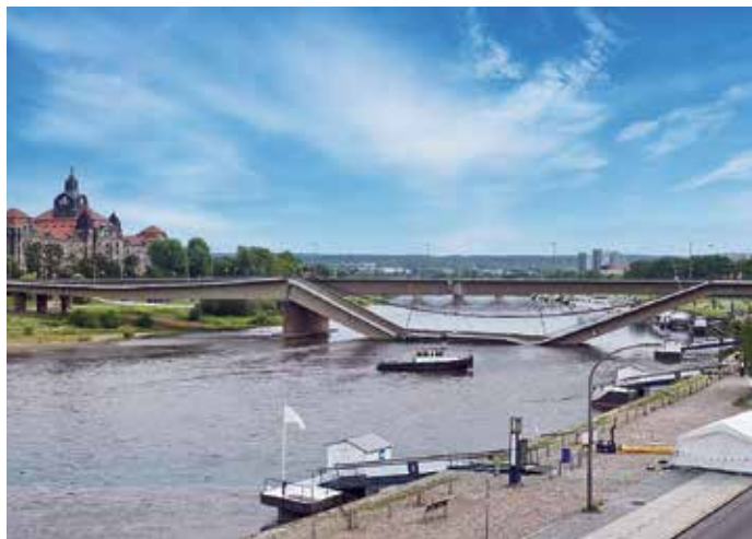
Photo: Collapse of the Carola Bridge on the River Elbe in Dresden, Germany, in September 2024. There were no fatalities, but significant disruption occurred, including the loss of hot water supply for the entire city and halting of shipping on the river. a formal investigation is ongoing but local authorities have stated that corrosion of steel reinforcement due to ingress of salt is likely to have been the cause of the failure.
