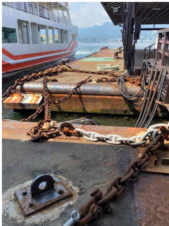
Photo 1: Shiny and Corroded Metal Chains (source: Private Collection).
