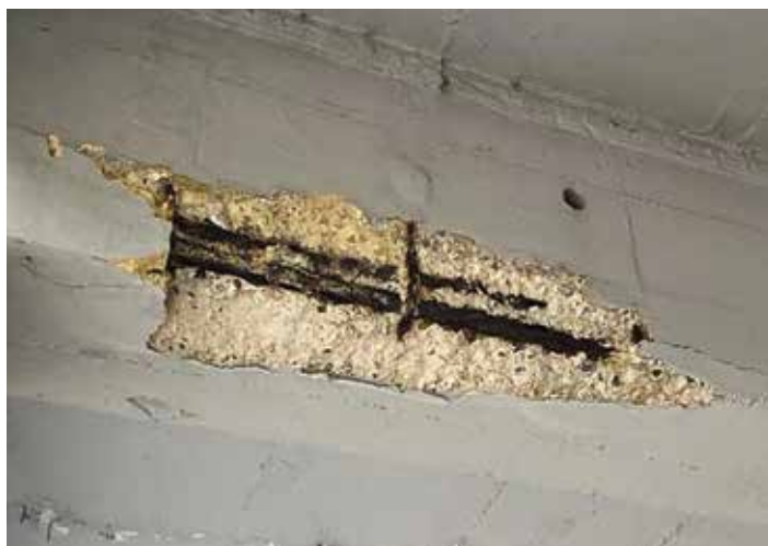
Figure 1: Cracking and Spalling Due to the Expansive Force Created by Corrosion of the Reinforcement (CPT).
