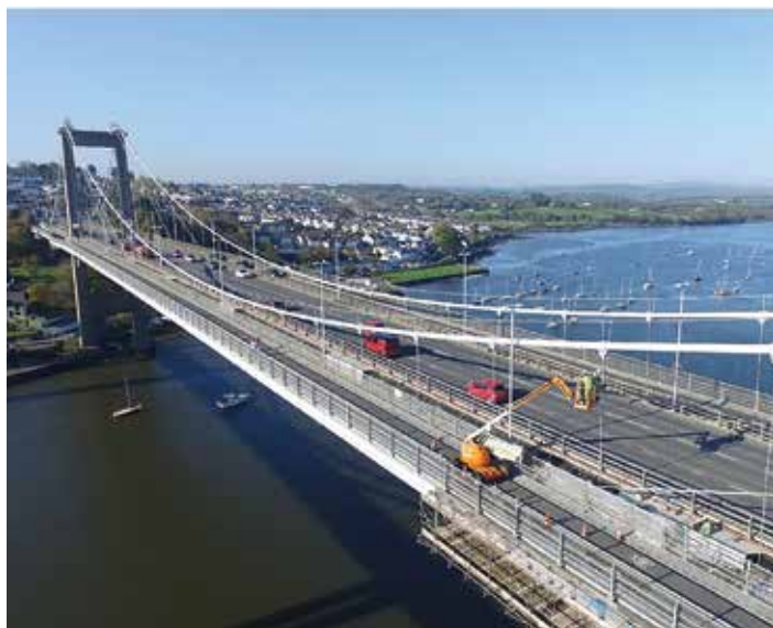
Photo: Overview of the Tamar Bridge With Cheery Picker Painting Maintenance Ongoing.
