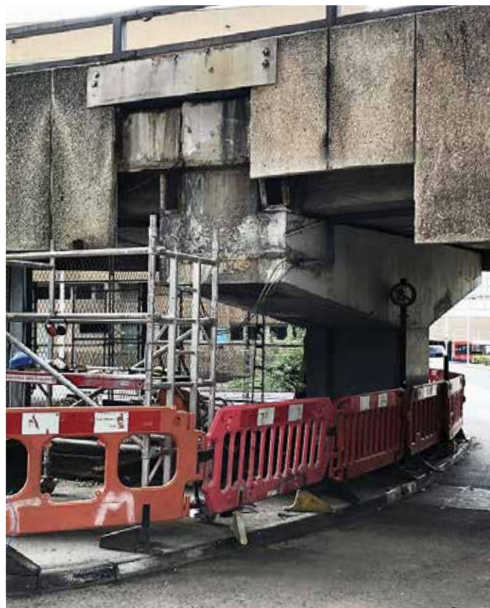
Photo: Trial Application of Concrete CAP on Bridge Crosshead at Coventry, UK.
