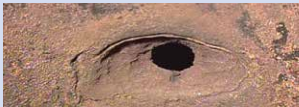
Photo: Pipeline MIC Corrosion.
