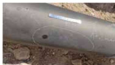
Figure 7 (a): Direct Examination Photos After Coating Removed and Pipe Blasting [1].
