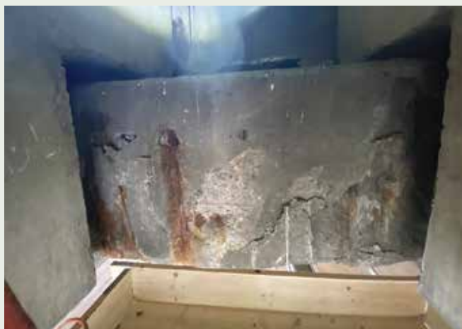
Photo: Crosshead Deterioration Between Beams M8 Woodside Viaduct, Image Courtesy of New Civil Engineer and Transport Scotland.
