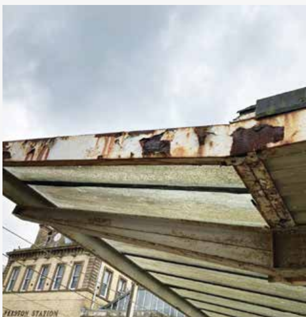
Photo: Spotted recently at Preston Railway Station, severely degraded coatings to Overhead Platform canopies, requiring urgent Fabric Maintenance.
