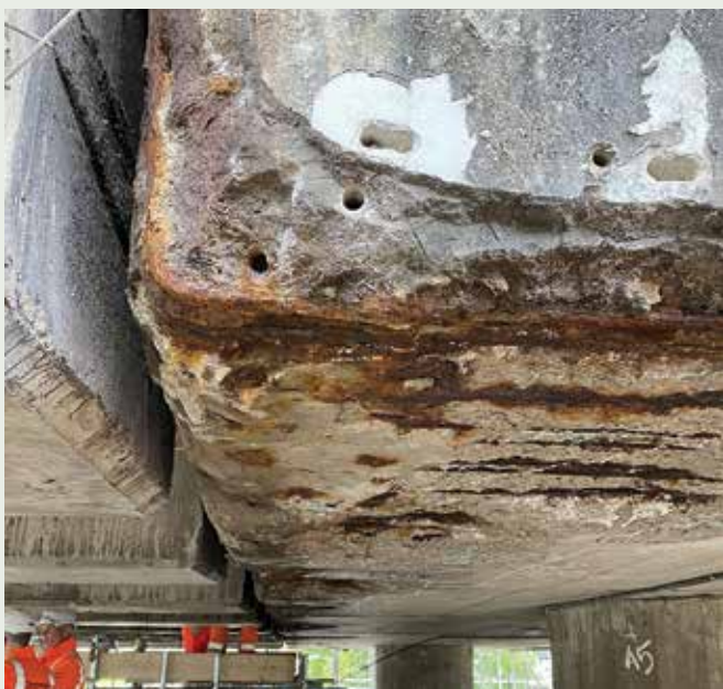
Photo: Reinforced Crosshead Deterioration at Deck Edge Eastbound Carriageway M8 Woodside Viaduct, Image Courtesy of New Civil Engineer and Transport Scotland.
