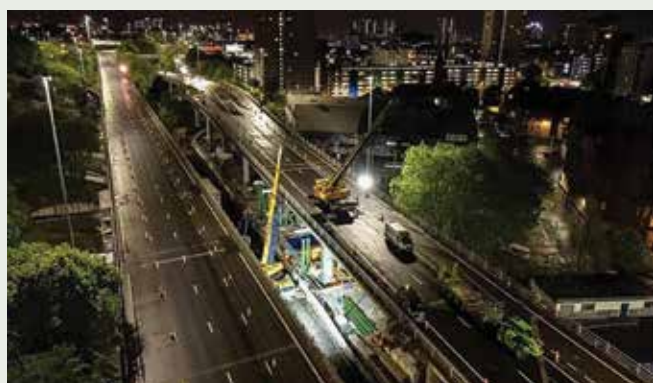
Photo: The Twin Elevated Woodside Viaducts Between Junctions 16 and 17 of The M8 Through Glasgow - a Critical Transport Artery Now Undergoing Major Corrosion Related Repairs, Image Courtesy of Transport Scotland.
