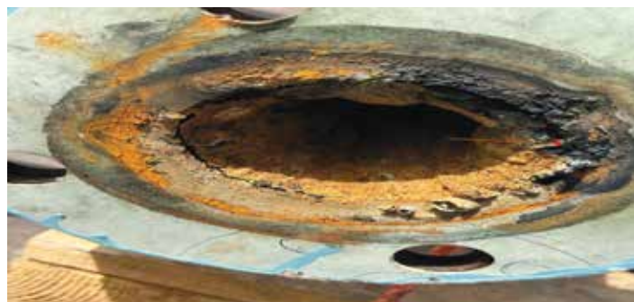
Figure 3: Deep Pitting Beneath Biofilm Layers.
