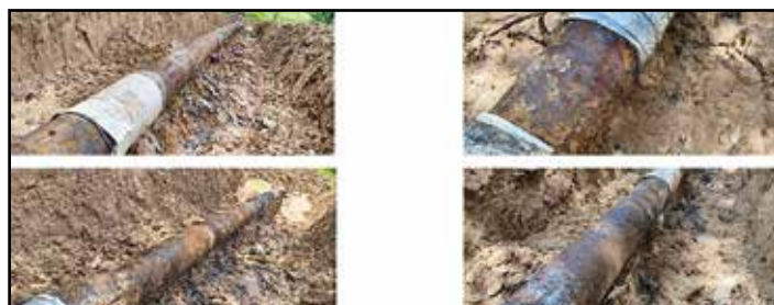
Figure 8 (a): Preliminary Sections of Exposed Pipeline Confirming Defects.
