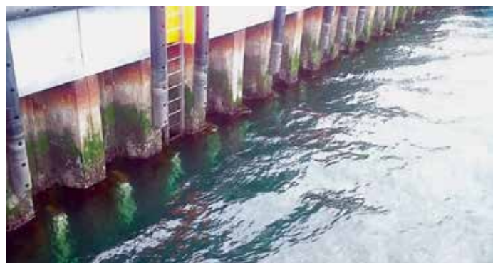
Photo: Monitoring of a Marine CP Installation.
