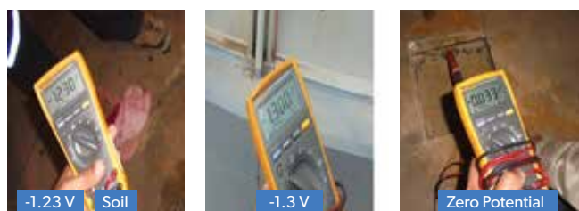
SS-T-Y Demin water tank CP measurement inside the tank
