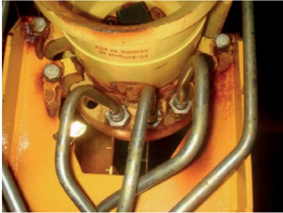
Umbilical connection showing severe corrosion(source: EEMUA Publication 194)
