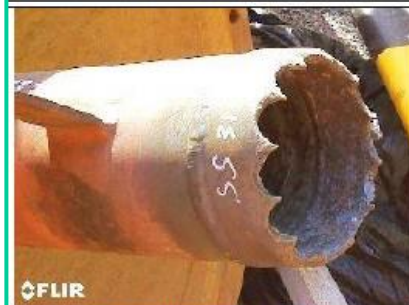
Figure 12C 7-F-0106; location-burner end cap; damage noted in high temperature corrosive combustion environment; existing material SS310; material upgraded to HR160- UNS N12160.
